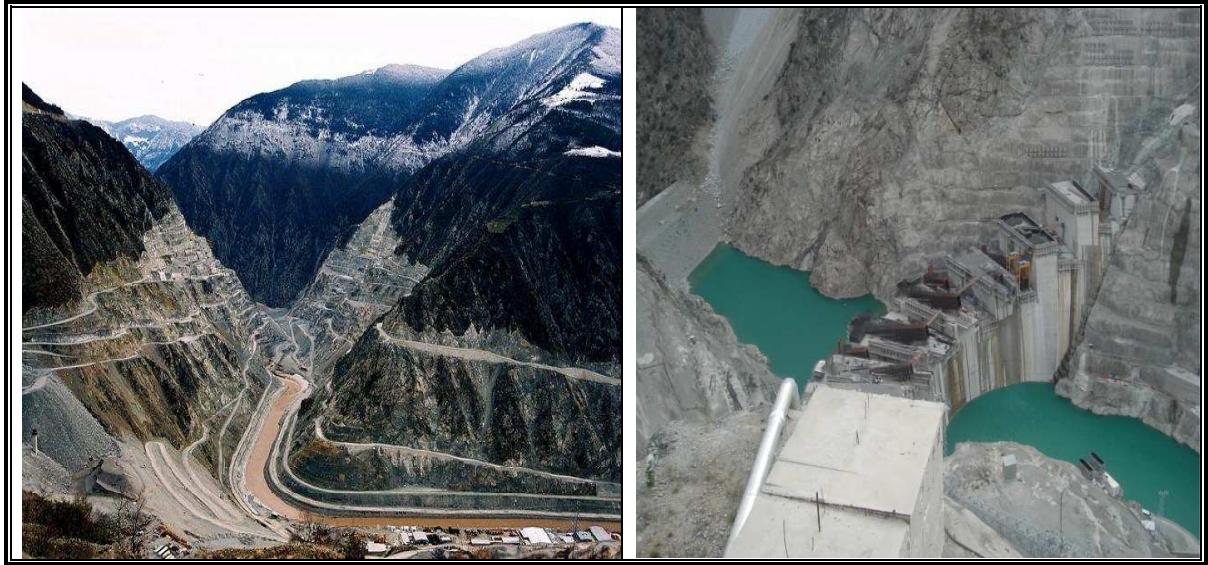
Figure 1: Deriner will become highest (247 m) dam in Turkey, it completed (Çoruh River-Artvin).
